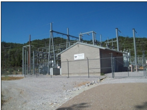
City of Shasta Lake Substation
