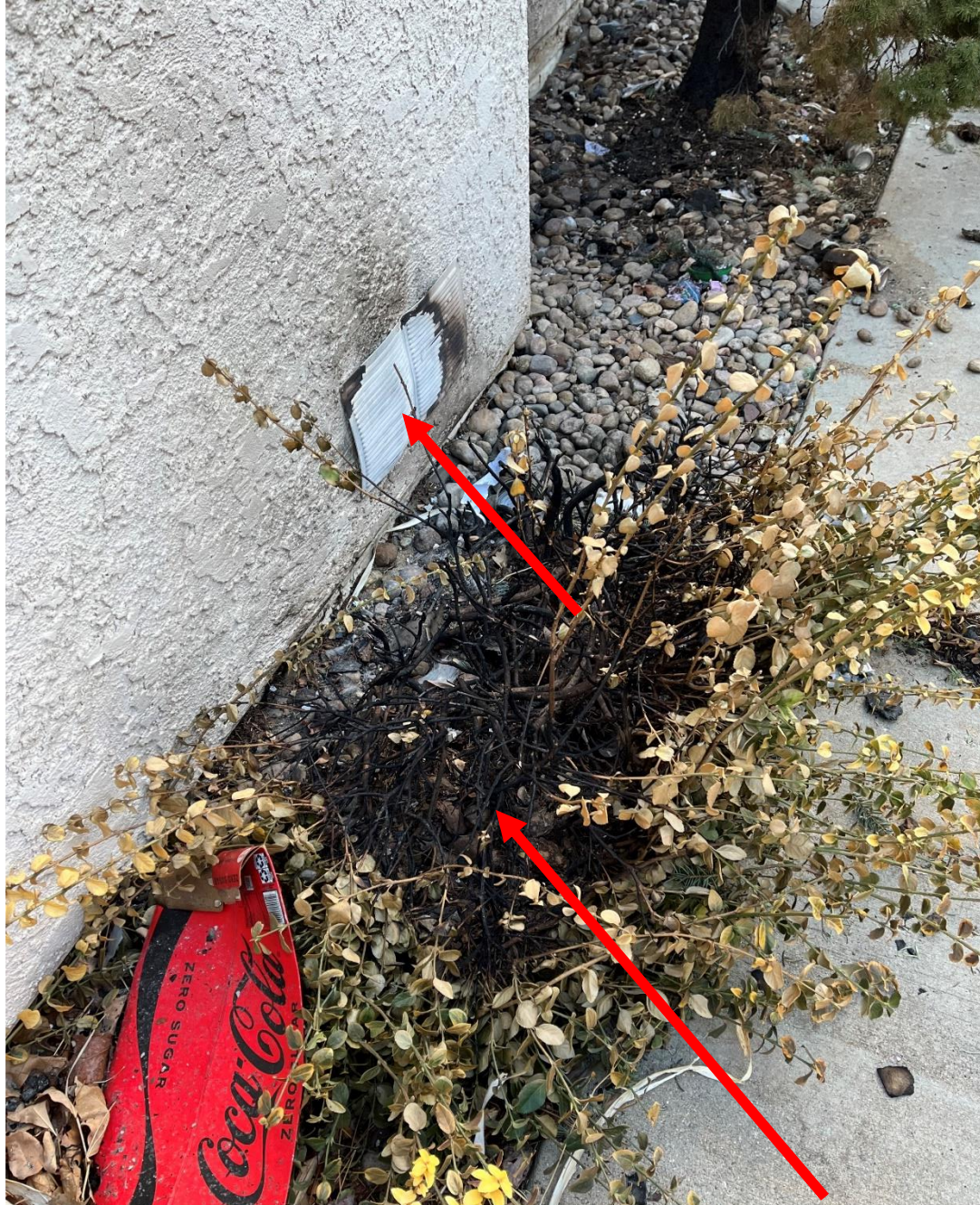
Embers to vegetation to vent
